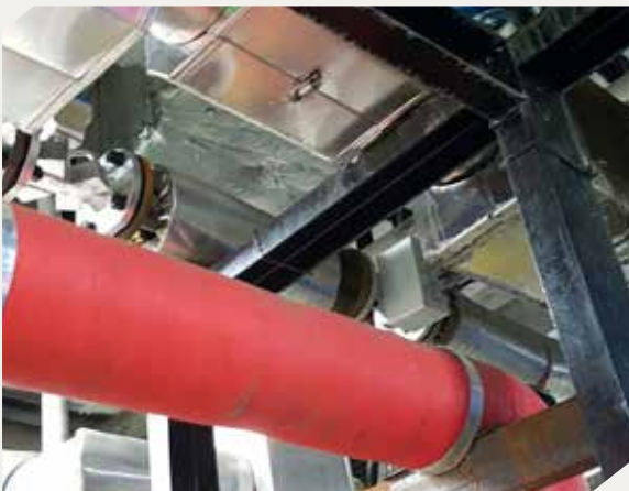
Korea District Heating Corporation (Xonic 10LE)
