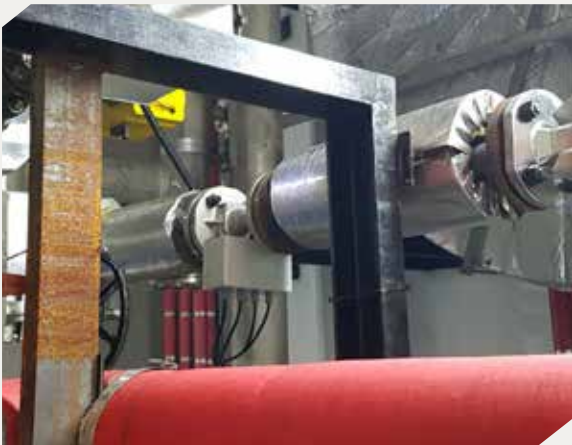
Korea District Heating Corporation (Xonic 10LE)
