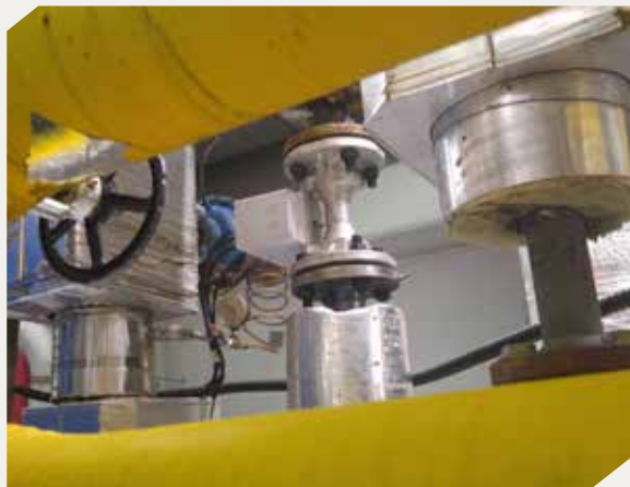
Korea District Heating Corporation (Xonic 10LE)
