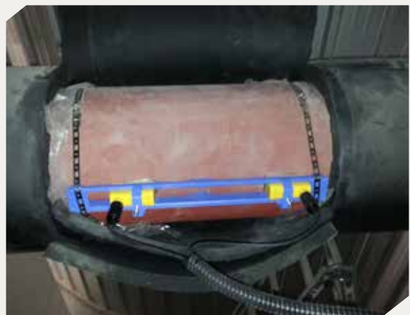
Daejeon City Eulji Hospital Ice Storage System (Xonic 100L)
